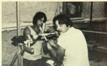
Shown in these two photos are the first cable-splicer graduates of Local 995, Baton Rouge, La. Here are Mike Schexnaydre, left, and Joe Aycock.
