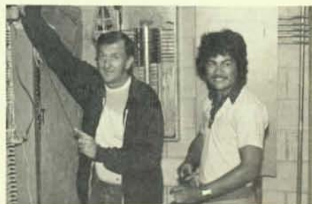
Brother J. H. West and Larry Josue are putting the final touches to a panel on a shopping center job.
