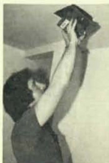
Executive Board member Dick Day of Local 46, Seattle, Wash., installs the fan in the you-know-where.
