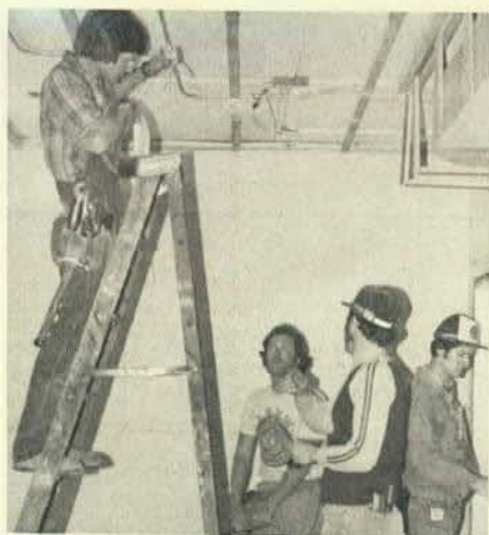
Shown here are Kennewick, Wash., second-year apprentices of Local 112 volunteering their labor to help remodel the old Pasco Library to be the future home of the Franklin County Historical Museum. From left to right are apprentices Brian Howard, Joel Harding, Jeff Patton and Duke Thietje.
