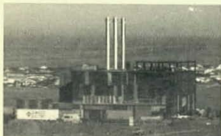
The University of Wyoming is building a new steam plant to better heat the rapidly expanding university.
