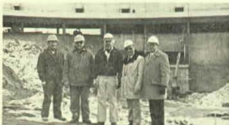
Left to right Brothers Dennis Motzko, shop steward for Sterling Electric; Herb Bremel, job steward; John Vitols, general foreman; Tony Mathiowetz, business agent of Local 292; and Jim Adams, president of Local 292, inspect the construction progress at the dome stadium in downtown Minneapolis. The wind chill at the time this photo was taken was 23° below zero.
