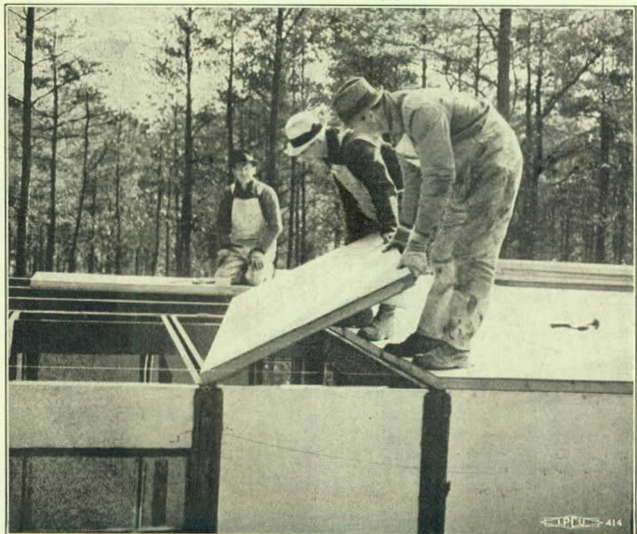
Workmen laying prefabricated slabs on a machine made house—a type which is not "taking hold" as this story indicates.
