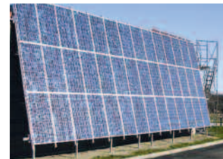
Solar voltaic installation at the Local 99 union hall in Cranston, RI.
