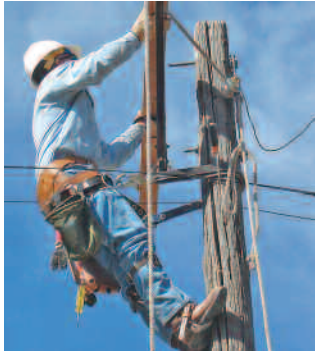
Local 667 lineman apprentice Scott Dougan works on a "reconductor" job out of the Canon City service center.
