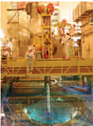
Local 245 members completed outages at the Davis-Besse nuclear power plant in Ohio.
