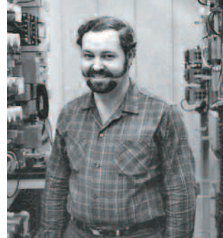
Local 547 Bro. Carl Foltz between relay racks in North Kansas City, MO, in the 1970s.
