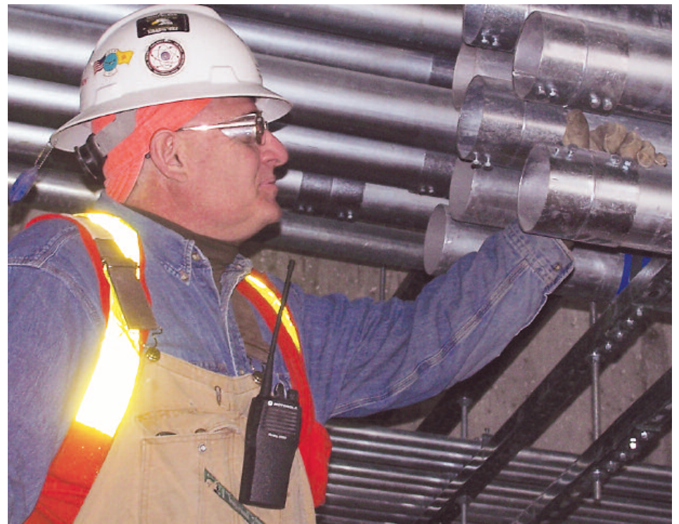
Denver Local 68 journeyman wireman James Keating checks a conduit run at a Code of Excellence project at Children's Hospital.
