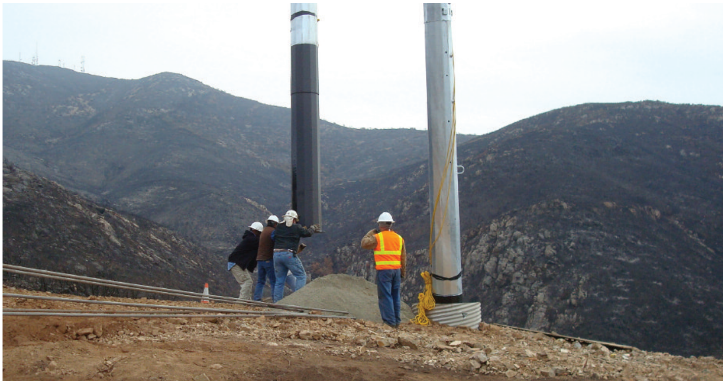
IBEW members on a crew from Diversified Utility Services set a transmission pole on Mount Miguel, in Chula Vista, with the assistance of a helicopter.
