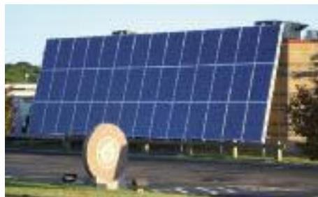
IBEW Local 99 hosts Rhode Island's largest photovoltaic system at its local union headquarters.
