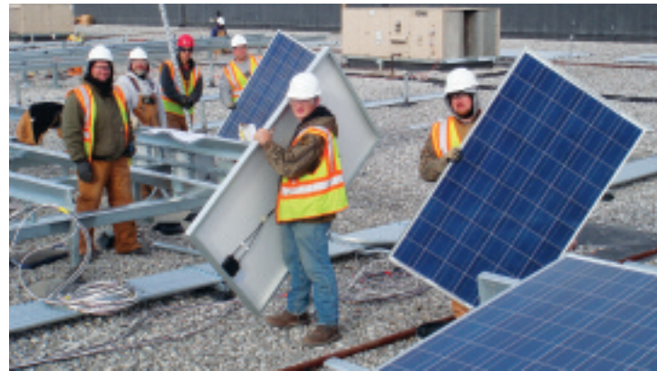
A York, Pa., Local 229 composite crew installs solar panels at Kohl's department store in Hanover. Journeyman wiremen Shane Reese, left, and Bob Cidor are joined by apprentices Klinton Kohler, Wes Copenhaver and Chase Stewart and construction wireman Ron Hilbert.
