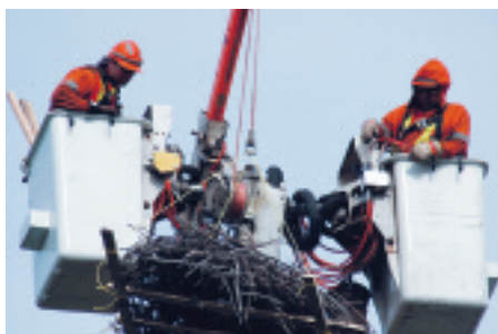
Local 636 members Brian Martin and Randy Kirkwood (Waterloo North Hydro) feather the controls as they help establish a new home for some feathered friends in their community.
