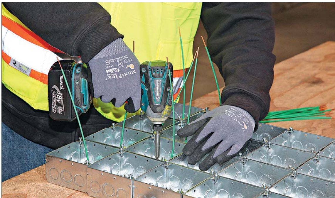
Working in climate-controlled prefab facilities, IBEW members are helping reduce construction time and costs, enabling contractors to get the jump on new projects.
