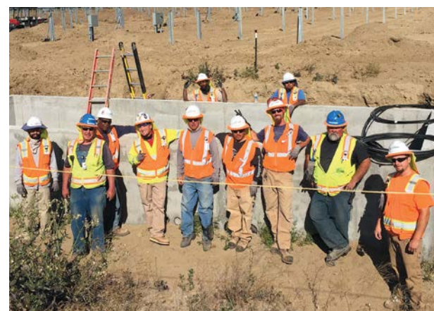
Working on the North Star Project are D/C feeder crew members from Local 100: general foreman Bob Grimes, foreman John Stevens, Darryl Stokes, Mike Chacon and Ellis Howard. They are joined by travelers from Locals 440 and 357.
