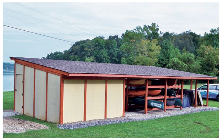
A new boat shed stands on the shores of Chickamauga Lake thanks to the hard work of union volunteers.
