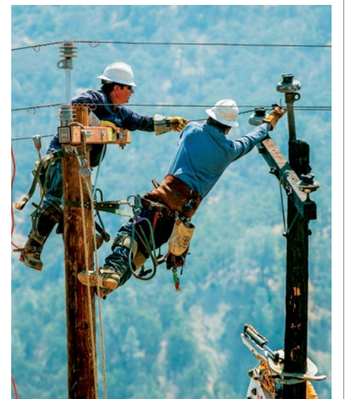
IBEW Local 1245 members Hollis Hadley (left) and Don Lee from PG&E replace a power pole that was destroyed by the "Rocky Fire" in Clearlake, CA.
