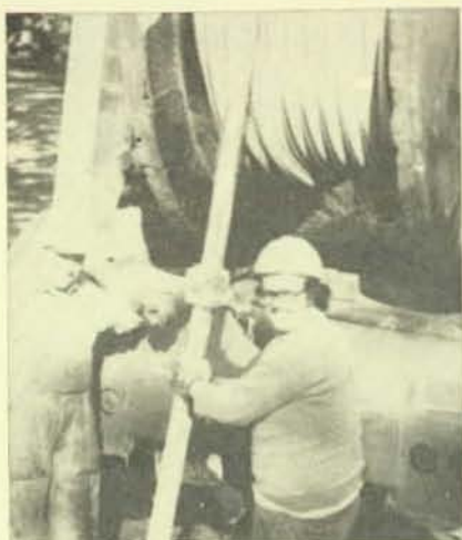
These scenes show members of Local 103, Boston, Mass., working on jobs. Here, Bill Caffavella and Frank Davey apply wire lube to 3-by-800 cable.
