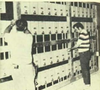
Brothers John Howland and Joe Monday, Local 728, Ft. Lauderdale, Fla., are pictured working on a dimmer bank on the Diplomat Hotel addition.
