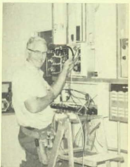
Brother Irv Sorg works on the power installation for the new IDRS computer system at the IRS Center.
