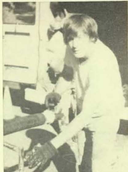
Brother Roger Sullivan installs pulling-eye on cable. This installation is the new primary feed to the new University of Massachusetts in Dorchester.
