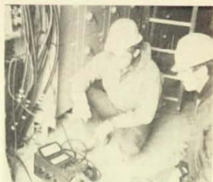
Members of Local 668, Lafayette, Ind., are doing the electrical work on the Eli-Lilly and Company's Tippecanoe Laboratories project. Here, checking the building feeders with a megger are Jerry Robertson, left, and Jim Brooks.
