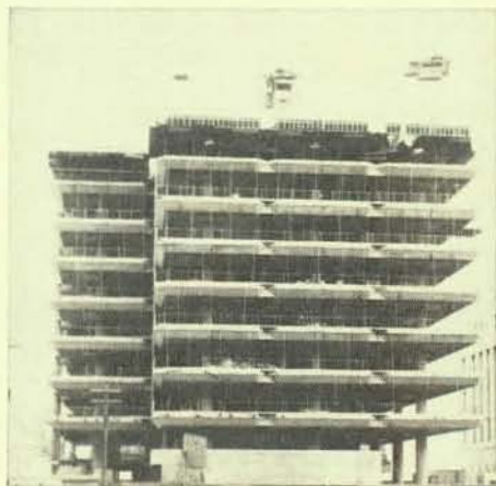
Shown is one of the three towers of the new $36-million home of the Bank of Canada.
