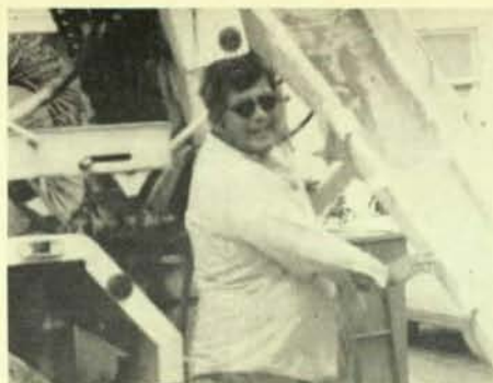
Members of Local 728, Fort Lauderdale, Fla. are working on the oil static job. Here Howard "Head" Fields is shown pouring concrete on the oil static job.
