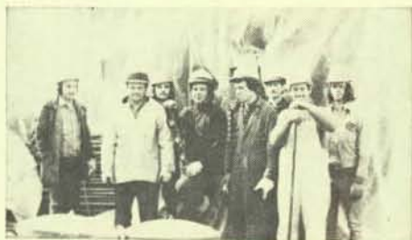
Brothers of Local 586, Ottawa, Ont., working for G. M. Guest, Ltd. are installing underground cables for Ontario Hydro.
