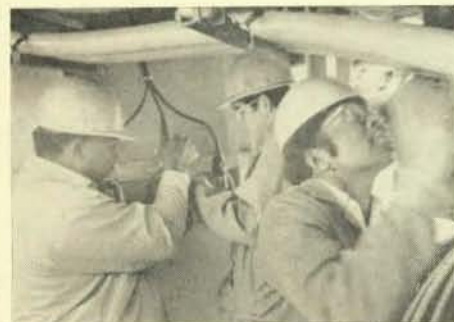
Connecting electronic equipment on board ship are Tetea Crum, Jr., left, an electronics technician who has been with Ingalls for seven years. Bobby Hicks, an electrician with the company for seven months, and Early Mumford, Jr., an electrical inspector with Ingalls for two years, are also shown. country, Ingalls is in a very good position for future business in the booming commercial shipbuilding industry."
