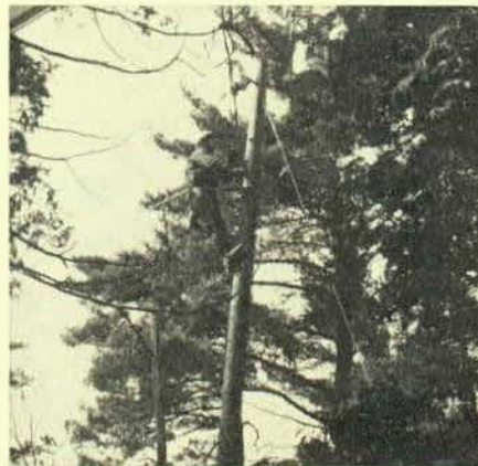
Brother Vic Barber changes transformer in low six point. The job is by Green Mountain Power Corporation, in a section of North Ferrisburg, Vt.
