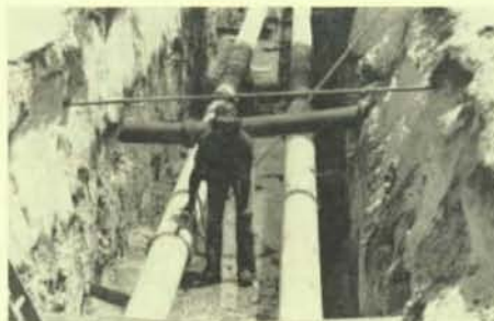
"Jeeping" the line. Electronic device is used to detect leaks in pipes.
