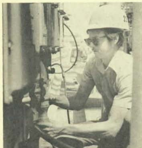
Michael Stokes, an electrical apprentice with the shipyard for one year, connects a cable from a newly launched ship to a dockside power supply to supply on-board power to the ship.
