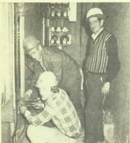
Working on electrical panels are Brother Charles W. Crossman, and in foreground, apprentice Brother Walter Hazelgrove, Jr. Looking on at right is Brother W. George Lester, who is in charge of this job for Northside Electric Company.
