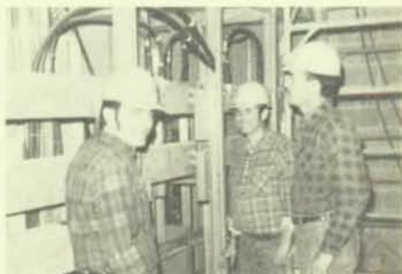
Brothers Cliff Batson, Richard Clarida, and Marion Moore are wiremen on General Telephone job at Carbondale.
