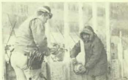
Brothers Gary Herren and Russel Miner wiring a swimming pool at SIU.
