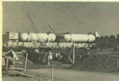
Left of the tanks are living quarters. At right is the refrigeration system.
