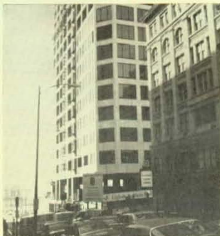
Eighth and Main building under construction in Richmond, Virginia on which members of Local 666, Richmond, Va., are working.
