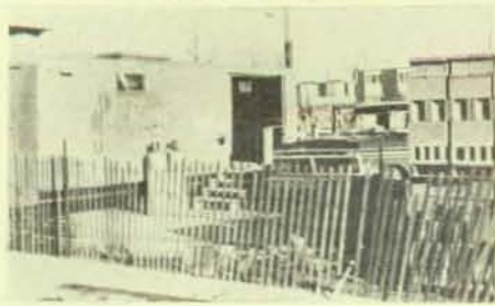
Scab construction site showing Parish trailer which is ABC. This is in the area of Local 665, Lansing, Mich.
