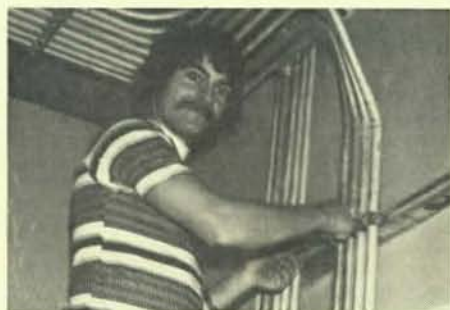
Quick Karl Butz straightens a pipe or two at the new VA Hospital, nearing completion in Boise.
