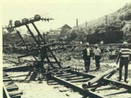
Here are scenes of the Johnstown flood with members of Local 459, Johnstown, Pa., helping to repair the damage. This scene shows Johnstown crews preparing to restore service to Bethlehem Steel.
