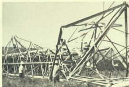
Members of Local 17, Detroit, Mich., are working on the damage wrought by a tornado in New Haven, Mich. The Brothers are foreman Dick Kille, Jerry Dixon, Jim Dunn, Jerry Woodruff, and Paul.
