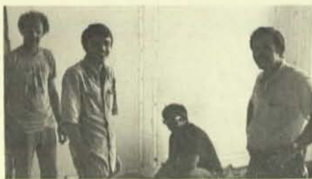
The hotel room renovation gang consists of George Fenwick, Pete Ireland, Joe Lombardi, and foreman Bill Cannon.
