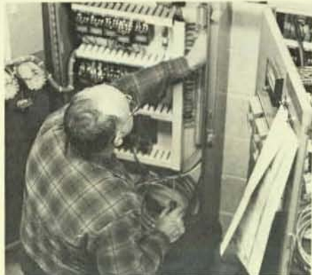
Brother "Pete" Hastings hooks up one of the many panels on the highly automated sewage treatment plant for the City of New Orleans.
