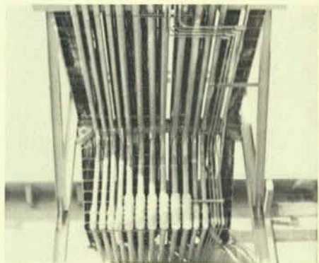
Shown is only one of the many conduit and cable tray racks installed by Local 505's members.
