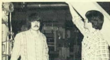
Apprentice wireman Dave Renner and journeyman wireman Jim Bryan working for McJohnson Electric at World Color Press in Salem, Ill.
