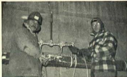
Brothers Charlie "PeeWee" Ernst and Tom Floyd of Local 369, Louisville, Ky., install heat trace at a local chemical plant.
