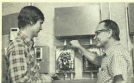
Greg Feimster, left, and foreman Eddie Moore are employed by I.K. Electric Company and are checking out the control system on the equipment floor at the Orbit Valve Manufacturing Company Complex at Little Rock.
