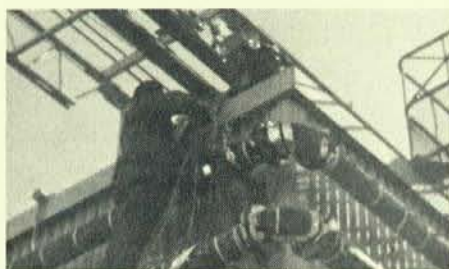
Brothers Don Collini, back to camera, and Kenney Hayes installing thermostats on heat trace system.
