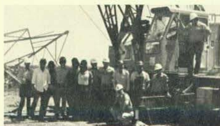
Left to right are Verne Peterson, Steve Say, Jim Dishman, Bernie VanPelt, Ron Holbrook, Scott Bean, foreman Slim Cargill, Bureau inspector Dave Rausch, Tex Montgomery, job steward Tom Huston, operator Scotty Strasser, Bear Osborn, and kneeling, Business Manager Ed Nicksic.
