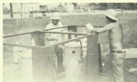
Don Welch, left, and Pat Irish installing a three-phase transformer bank in South Burlington, Vt. Is Pat reading a love letter or instructions?
