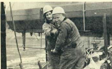
Roger Martin and Curley Shutter working at removing a cover from one of the 765-KV transformers.
