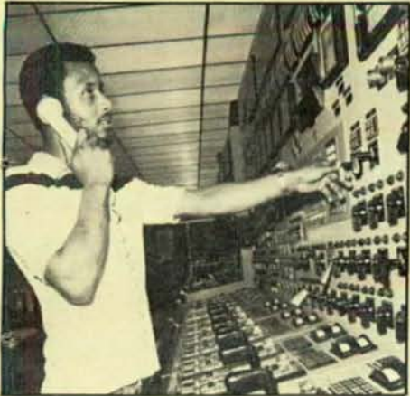
LU 2337 member David Williams, TUGCO assistant plant operator, is shown at the control panel of the Monticello steam electric station.
