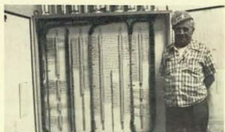
Brother Frank Shinall, Jr., of Local 68, Denver, Colo., is shown standing by the communications panel he completed on the Rocky Flats project. The cabinet contains a wide variety of scales and wire sizes, all quality controlled.
