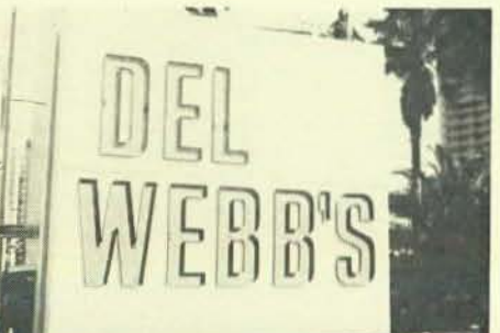
Doug Boyd, top right, installs brackets so that top of sign can be hoisted into place.
