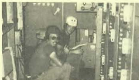
Joe Zeboski and John "Dago" Williams do maintenance work for Sipes Electric, Inc. at Morris No. 5 mine, Pittsburg, Ill.
