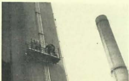
Working on the smokestack at Station 16 are Brothers Lanny Inman and Don Carlson.
