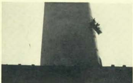
Working on the smokestack at Station 16 are Brothers Jim Morley and Rick Rottman.
