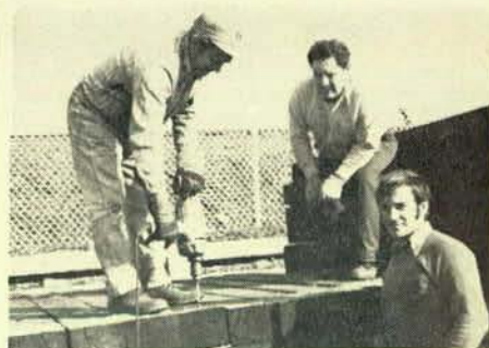
Preparing third-rail ties at the Maintenance of the Way Yard in Clifton, left to right, are Brother Joe Russo, drilling out the new ties; Brother Sparky Riccardella, third-rail foreman; and Brother Pete Argenziano, treasurer of Local 922.
