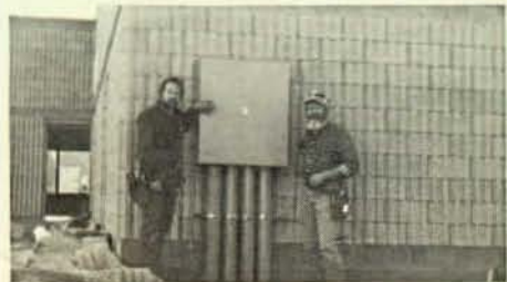
Shown are Bert Sargent and Pat Bacus standing by the new office building under construction for Local 322, Casper, Wyo.
