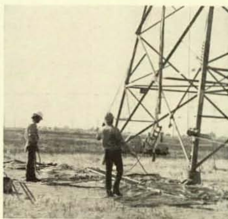
Readying mobile insulated boom to be hoisted up the tower are linemen Mike Eckhardt, left, and Dennis Jorgensen. (See Local 1245's letter for details.)
