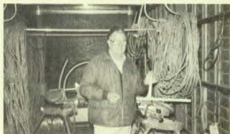
Lou Baumeister, also known as "Mr. Fixit," of Local 262, Plainfield, N.J., rigged up this BX cutter and stripper while at the Hilton Hotel at Somerset in Franklin Township, N.J.
