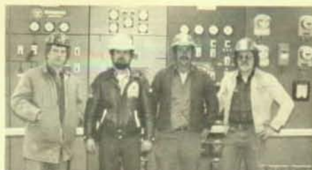
Left to right are Dennis "Red" Henderson, shop steward; Dave Chase, foreman; Brian Coburn, and Luc Chasse from Local 2166, Fredericton, N. B., in front of the 13.8-KV switchgears situated in the recovery boiler project in Atholville, N. B. These switchgears feed different parts of the mill.
