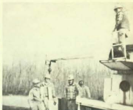
A crew of Local 702, West Frankfort, Ill., completes construction of two high-lines. Left to right are Alton Holtz, Scott Birkhead, Dan Kite, Scott Bradford, and Don Mangold.
