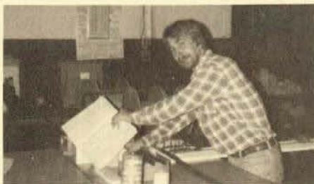
Brother Tom Kontz wires harness for Fincor Products, being done in Jno. Z. Barton's Panel Shop.
