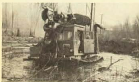
The swamp buggy is being operated by Illinois Valley Electric Co-op members to build 12-KV line near Hennepin, Ill.
