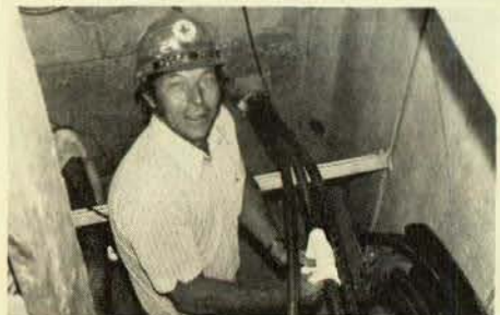
Rocky Owens, member of Local 76, Tacoma, Wash., working on manhole terminations at Satsop Nuclear Plant.
