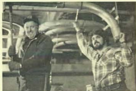
Installing conduit on hospital project are Joe McGrail, left, and Tom Joyce, members of Local 81, Scranton, Pa.
