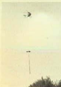
The approaching pole-setting rig typifies the vast changes we have experienced in the electrical industry in recent years.
