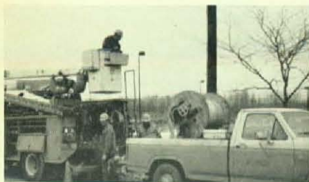
Pictured is the line crew on the Route 57 project, members of Local 79, Syracuse, N.Y., Bill Ryan, Ted Alletzhauser and Bill Helterline.
