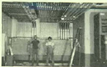
Pictured are Mark LaBlanc and Cory Qualls of Local 364, Rockford, Ill., with telephone and data conduit they installed at Sundstrand Aviation Plant in Rockford, Ill.
