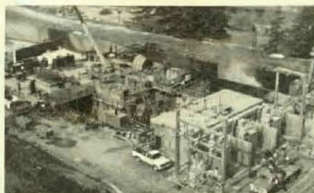
Pictured is the Friant Canal Powerhouse. It is one of three powerhouses at the Friant Dam being built with the aid of members of Local 100, Fresno, Cal.
