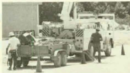
Pictured are line crew members of Local 398, Charleston, S.C., working on the Ashley Phosphate Road.
