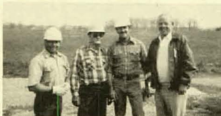
Pictured from left to right are Sammy Brooks, Nolen Kinkade, Bob Purnell and James B. Moore, business representative. These Brothers are part of the crew who are rebuilding the transmission line north of Benton, Ill.
