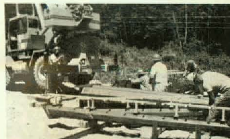
Shown is the Buffalo Electric Marcy-South job east of the Hudson River. Danny Dafoe's crew are prefabbing and setting the bottom sections.
