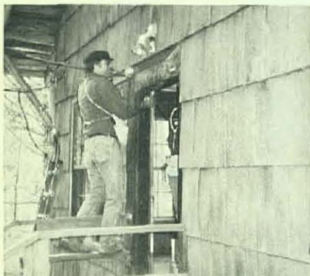
Local 280's business manager, Mike Murphy, traveled all the way from Salem to show Local 48, Portland, Ore., electricians some techniques of working during ladder shortages.
