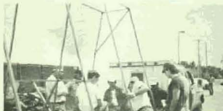
Brothers Dale McGarvie, Richard Garcia, Local 357, Las Vegas, Nev., Business Manager Cecil Wynn, Jr., Paul Yates, Joe Quercia, Stan Yuhas, and Ron Carter check out the strength of the trailer tongue of the first completed frame.
