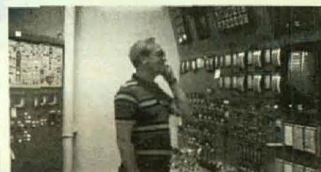
Pictured is Local 702, West Frankfort, Ill., member Paul Smith at the control board of Brown Station, Unit No. 2.
