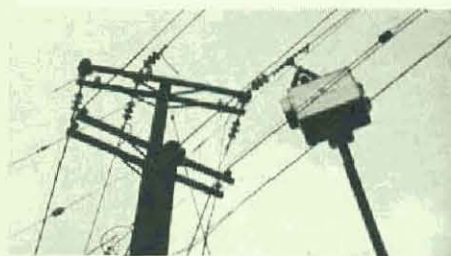
Local 70 members are shown at work on overhead distribution work for Riggs-Distler Company.
