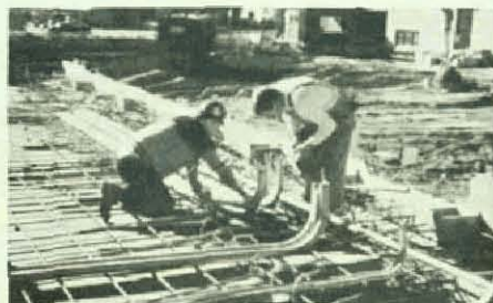
Brothers Curtis George and Terry Yorke are shown finishing conduit runs at the new Water Pollution Control Centre.
