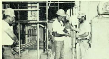
More of the Brothers who volunteered to repair damaged cables at the powerhouse jobsite are Dick Hall, Cliff Rouse, and Walter Snipes. (Photos submitted by Local 177, Jacksonville, Fla.)
