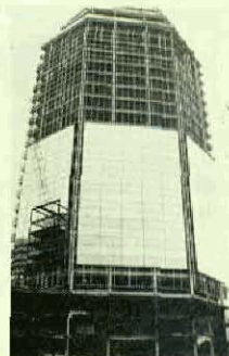
Pictured is the 26-story Monarch Tower. Collins Electric Inc. and Local 7, Springfield, Mass., are doing the electrical work.
