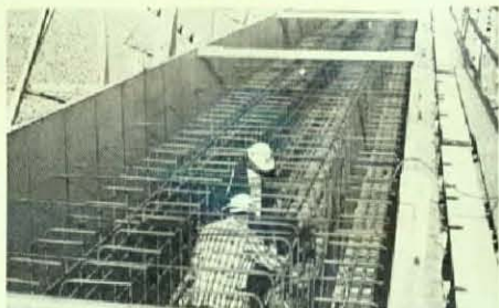
Pictured are Leonard Wright and John Williams cadwelding to rebar at the new Madigan Army Hospital project. This is the first pour of the 52-month project.
