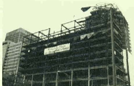
Also being built at the Monarch Place is the Sheraton Hotel, which is attached to the Monarch Tower. Monarch Place is the largest construction project in the history of Springfield.
