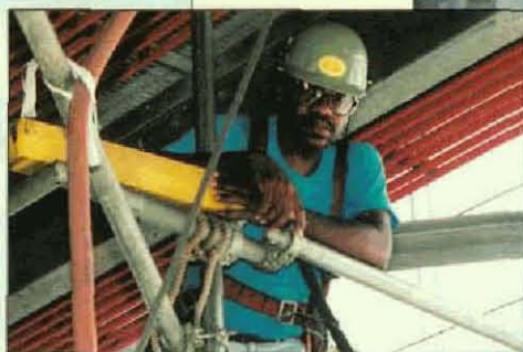
Above, Local 508 member Val Stephens prepares to operate an electric crane at the boiler complex.
