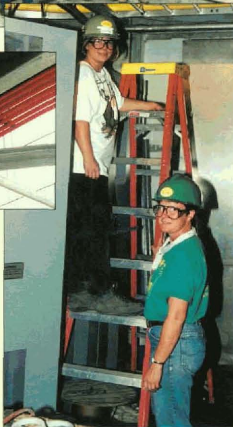
At right, Local 508 members Scarlett Hunt (left) and Sandra Brown (right) terminating cable into cabinets.
