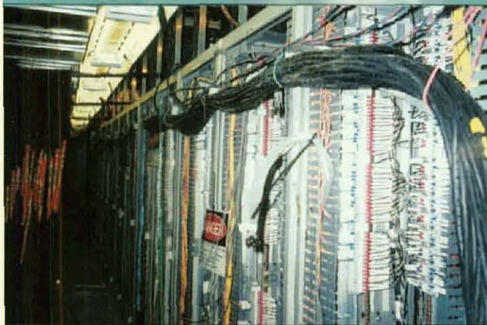
Above, some of the complex electrical wiring IBEW members have been doing for the recovery boiler project.
