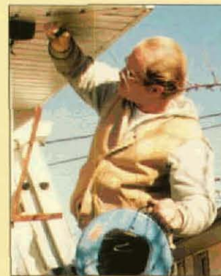
Local 354, Salt Lake City, UT, journeyman Van McAlister wires a security light for an elderly homeowner.
