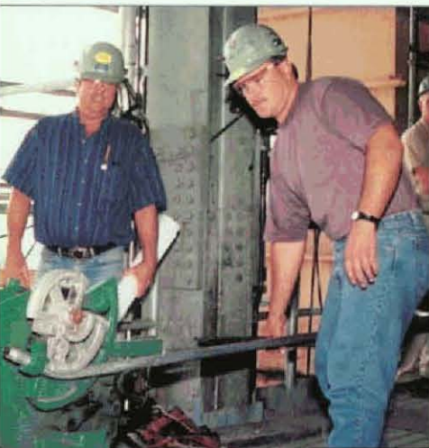
Above, Foreman Rick Canady (left) observes Local 508 member Creig Self bend conduit.
