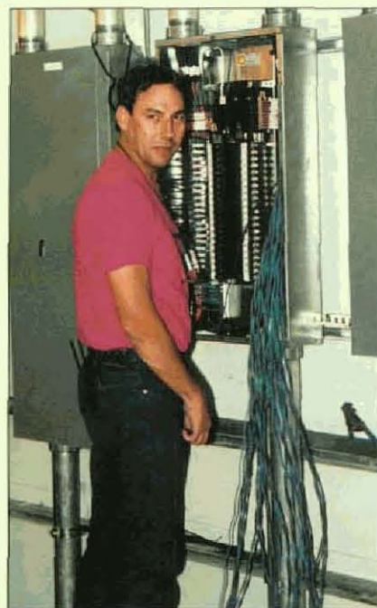
In the Rack Room, Local 508 member Ralph Harris hooks up and labels wires coming into a control cabinet.
