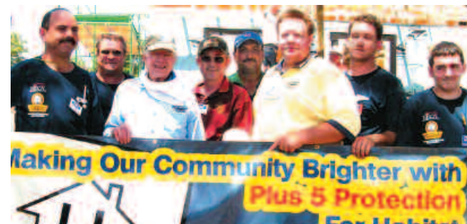
Local 153 hosted a 20-house blitz build for a Habitat for Humanity "Jimmy Carter Work Project." Some 180 IBEW volunteer wiremen included members from sister locals as well as Sixth District international representatives. Pictured with President Jimmy Carter (third from left) are, (L-R): Jerry Talamonti, Local 127; Ralph Rose, Local 127; Jim Dudley, Sixth District residential organizing coordinator; Local 153 Bus. Mgr. Mike Compton; Sixth District Int. Rep. David J. Ruhmkorff; Mike Fenrick, Local 153; and D.J. Constable, Local 153.
