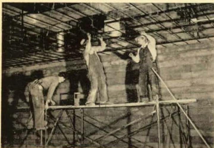
L.U. 6 members Ralph Hill, Jesse Mendez and Frank Jovich install loud speaker system circuits in new Emporium Department store located in big Stonestown Housing Project.
