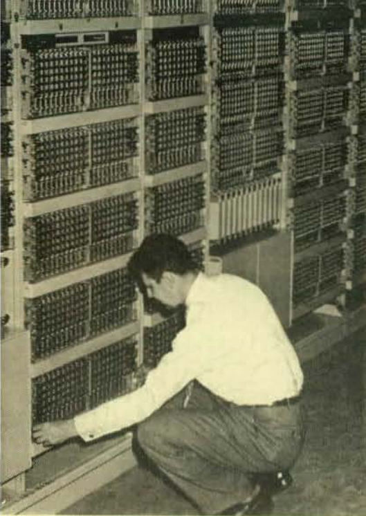
Larry Lucas checks select bar on line link frame of crossbar switch.
