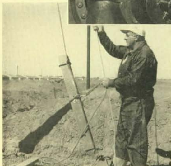
Tom Barr, groundman, sends up a cross-arm to his working partner on a pole as power lines are extended by members of 1245 to new development.
