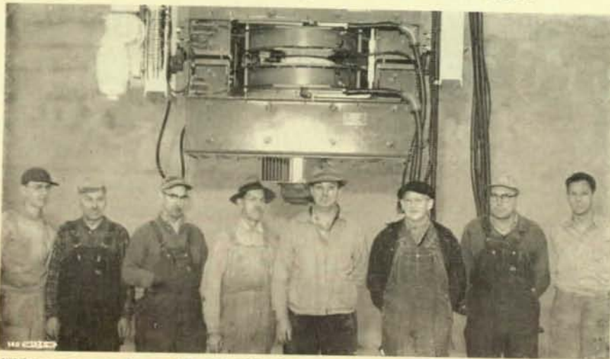
This crew, members of L. U. 654, Chester, Pa., installed this betatron, a giant x-ray machine, employed in the inspection of welded tank components. They are, left to right: R. McBride; S. Hoeffler; J. McBride; J. Dean; H. Frank (General Foreman); F. Horne; H. Sheppard; and J. Hoeffler.
