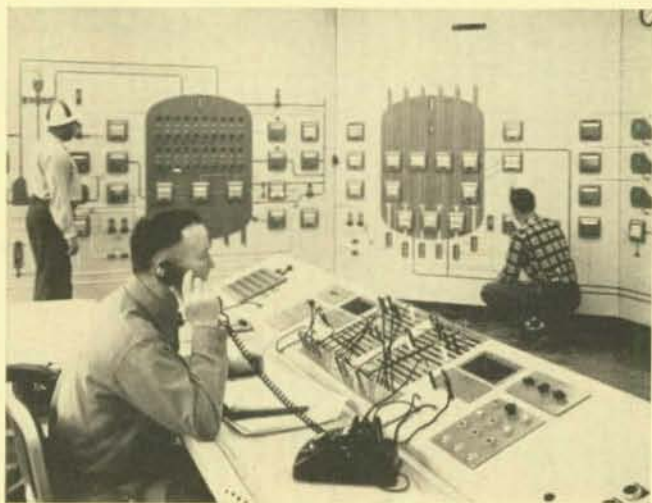
Ultra-modern control board of the catalytic cracking unit has a plug board, at center, which permits read-out of any point on console digital indicators.
