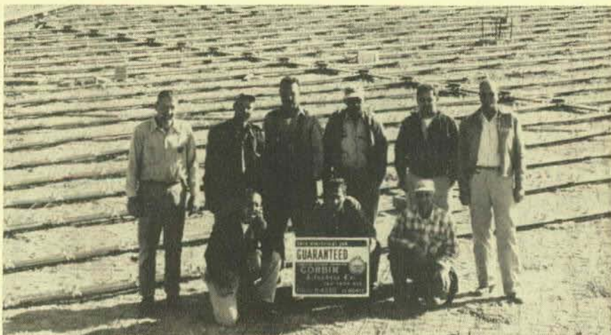
More than 18,000 feet of underfloor fiber duct has just been installed by these men of Local 11 in the new engineering building of Aerojet General Corporation of Azusa, Calif.
