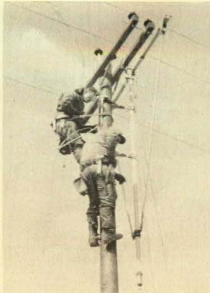
Brothers Harold Eastwood and Doyle Lamb of Local 196, Rockford, Ill., installing set of double, 8 foot arms on 3 phase line with hot line tools.
