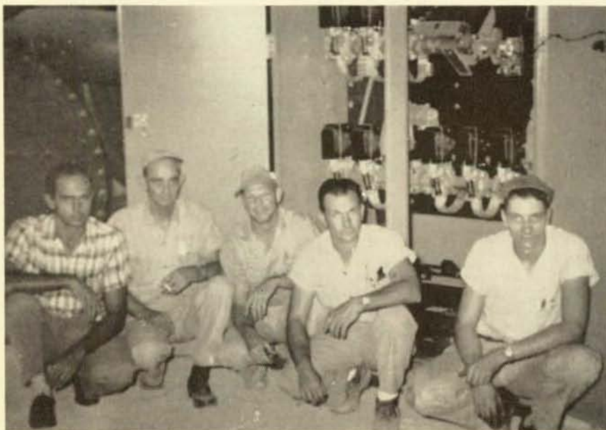
Starter located in Chemistry Building, University of Alabama to control 400 HP Compressor. From left to right: Slim Stewart; T. E. Brazeale; E. R. Waites; C. W. Worthington, foreman, and J. A. Ball. They are members of Local 136, Birmingham, Ala.
